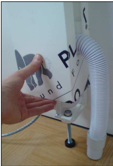
Feed leg cover up from underneath the sink on the left hand side, feed armoured cable and flexible waste through the slots and lower the cover down.
